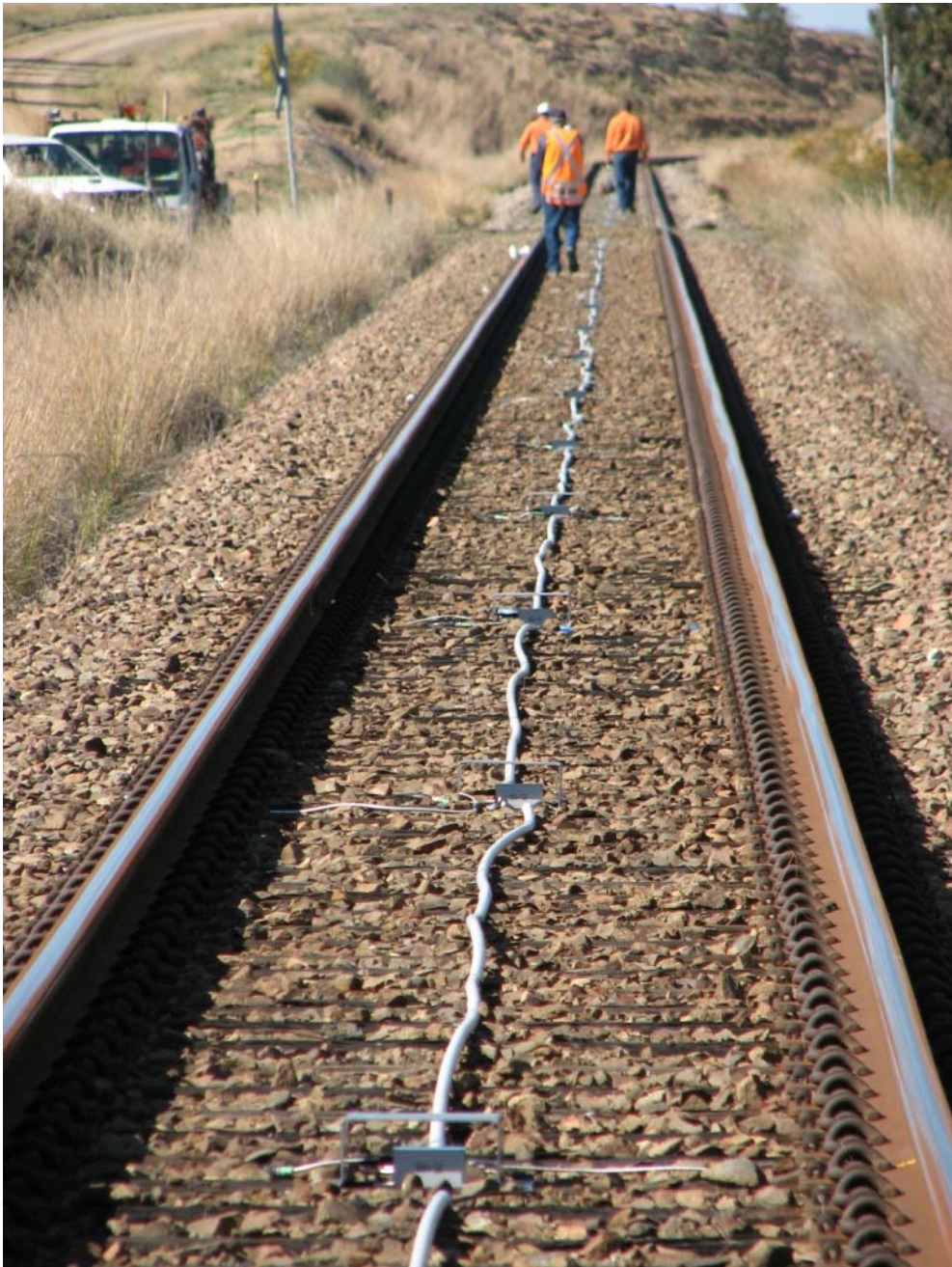
Figure 3 - Sensor installation along railway
